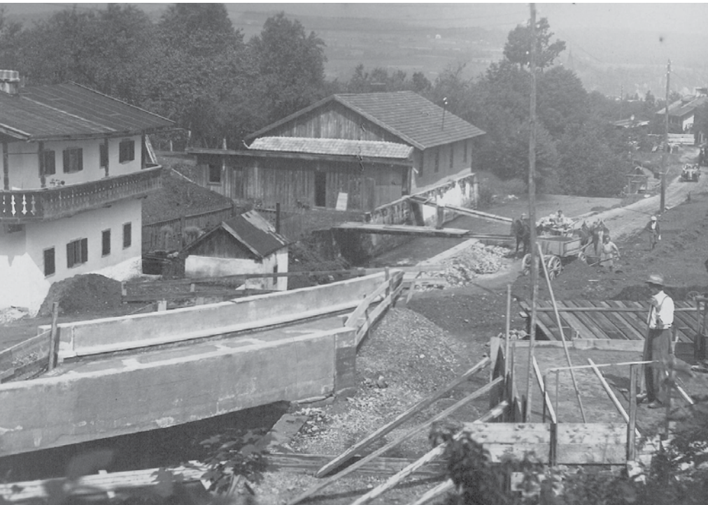
The new bridge under construction as part of the Miracle of Wörgl .
